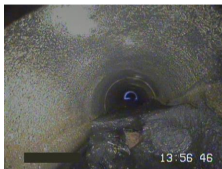
...deposits at the bottom of the pipe
