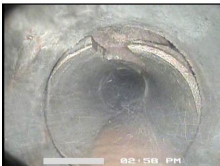
...localized pipe damage
